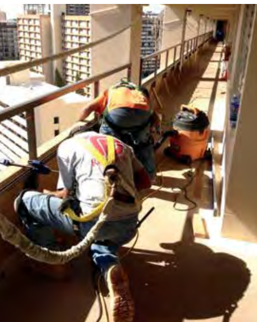
A recent balcony repair by Structural Systems PHOTO COURTESY STRUCTURAL SYSTEMS INC.
