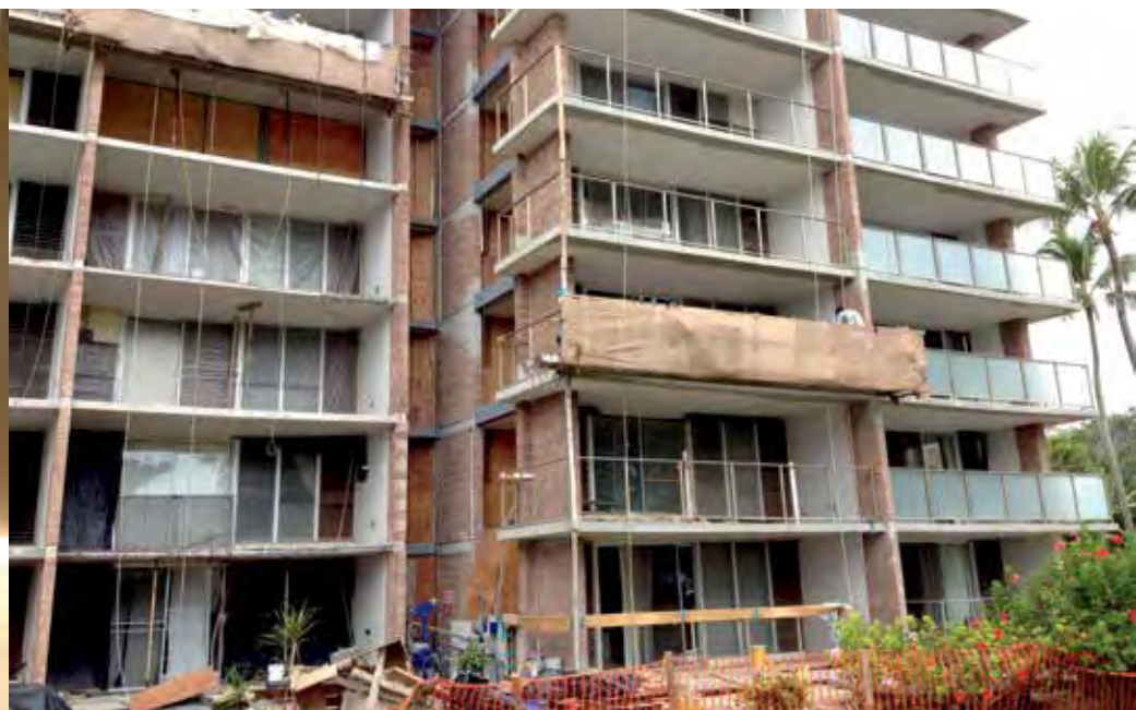
A recent concrete deck and railing repair by Structural Systems PHOTO COURTESY STRUCTURAL SYSTEMS INC.
