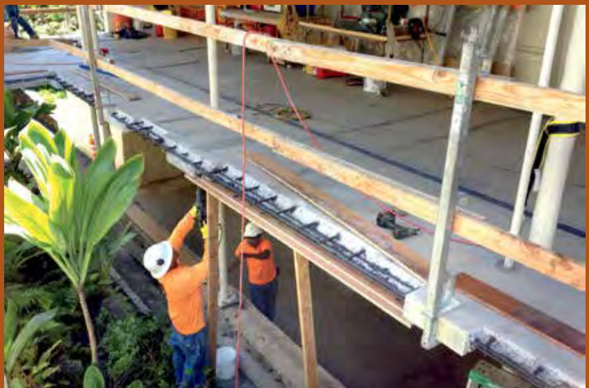
A recent deck repair by Structural Systems PHOTO COURTESY STRUCTURAL SYSTEMS INC.
